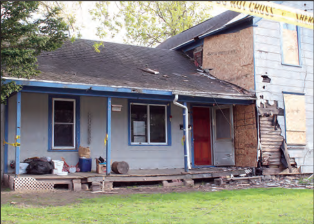
One person died in a house fire on East Center Street in Shawano the evening of May 6. KEVIN PASSON | NEW MEDIA
