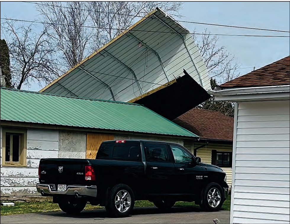
A metal garage was blown over on its side atop another roof in Mattoon.
