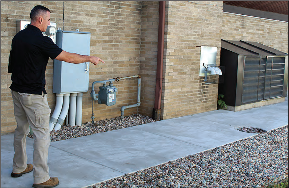
Grant Bystol, Shawano County highway commissioner and a member of the county's ad hoc building committee, points to an area his staff repaired on the north side of the Shawano County Library. The committee will eventually recommend a course of action regarding the library, courthouse, jail and sheriff's department — to continue the existing maintenance plan, renovate or build new.
