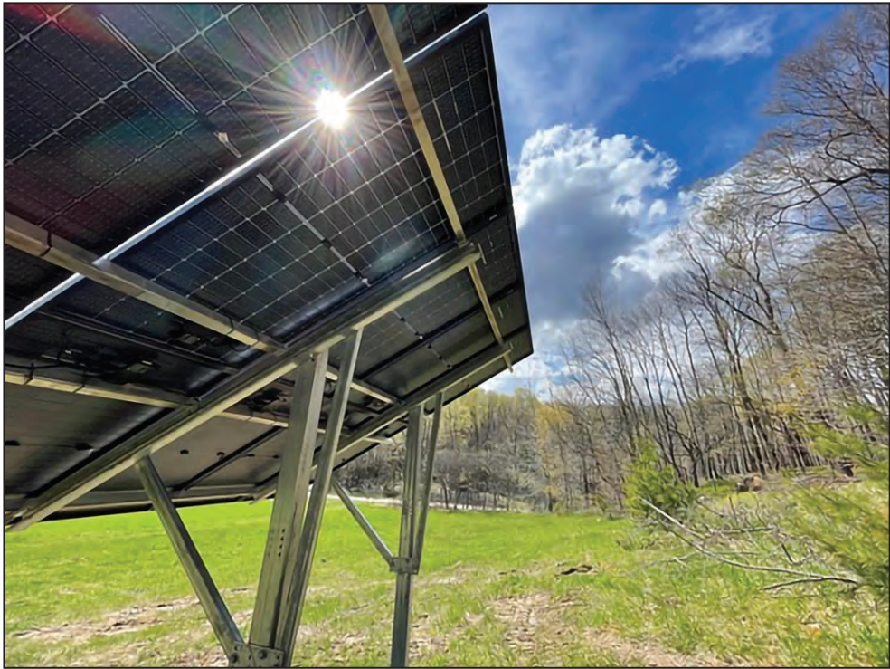
A newly installed solar array stands in a field in Marion. This small array will save a local cabinet manufacturer $981 per year, replacing 89% of the company's energy use.
