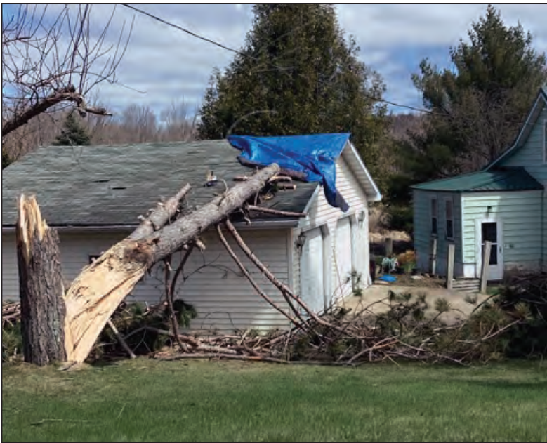
Damage to homes, trees and utility poles were reported when a tornado with estimated peak winds of 80 mph struck Mattoon on April 28. Minutes before, another tornado was sighted east of Birnamwood.
