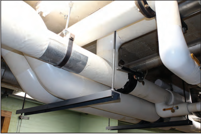
Repairs to heating pipes can be seen in the behind-the-scenes areas in the basement of the Shawano County Courthouse. The county has created an ad hoc committee to study whether to continue to maintain county facilities, remodel them or build new.
