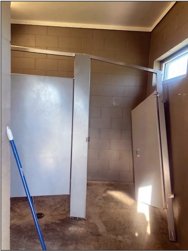
A stall door in the restrooms at Smalley Park was damaged recently, one of a number of vandalism incidents in Shawano's public parks. CONTRIBUTED
