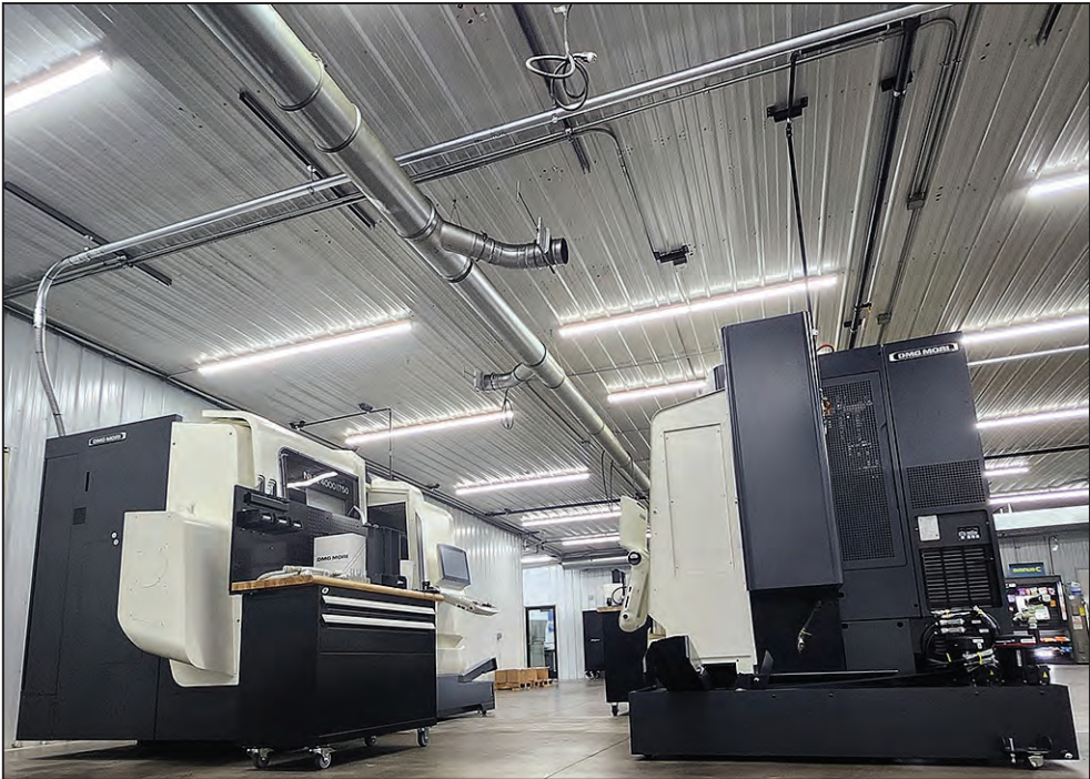
The installation of two DMG MORI NLX 4000 CNC turning centers is expected to be a game changer for JR Machine in Shawano. CONTRIBUTED
