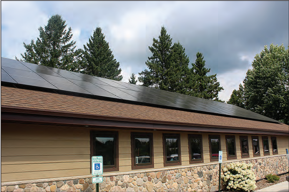
Solar panels were recently added to the roof of Lakes Country Public Library and will help to lower the costs to keep the lights on for patron visits and the many activities taking place within the building.
