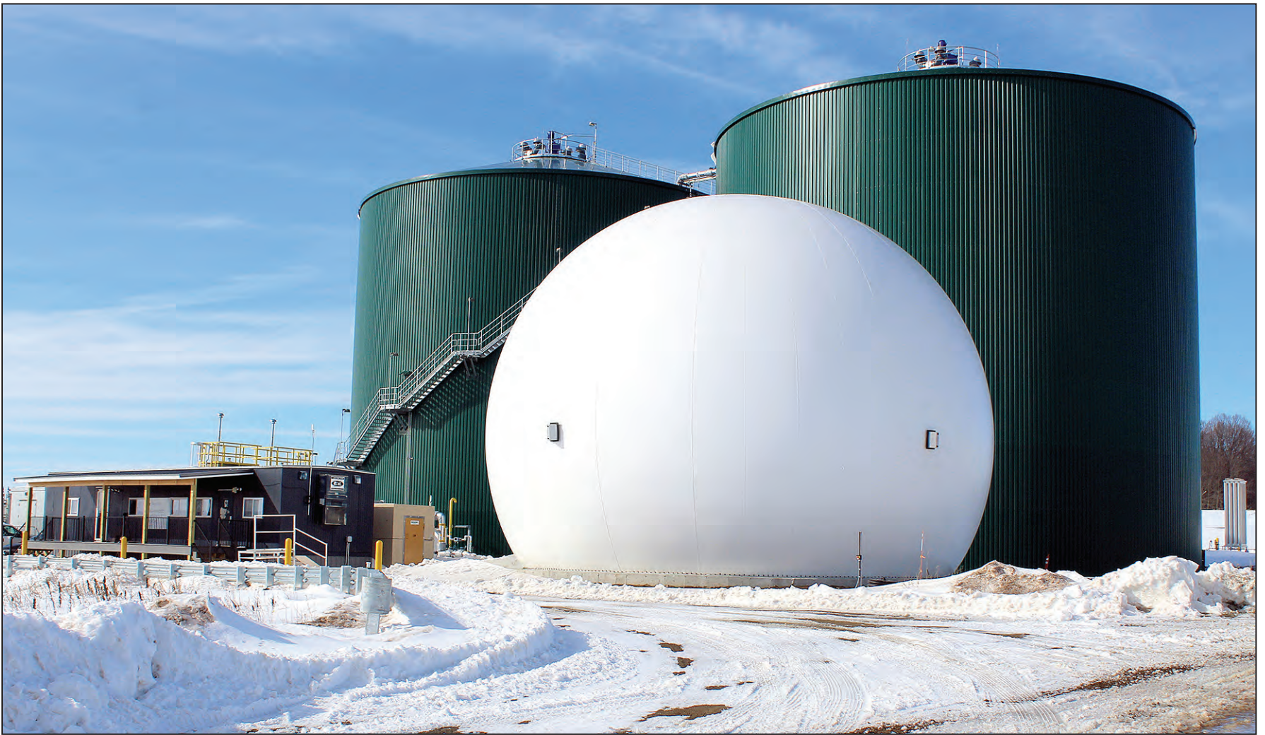
Tanks and snow sit on the DTE Vantage facility near Matsche Farms, Inc. in Birnamwood. The biomass processing plant opened last month and takes waste from Matsche cattle and turns it into natural gas for use in vehicles out in California.
