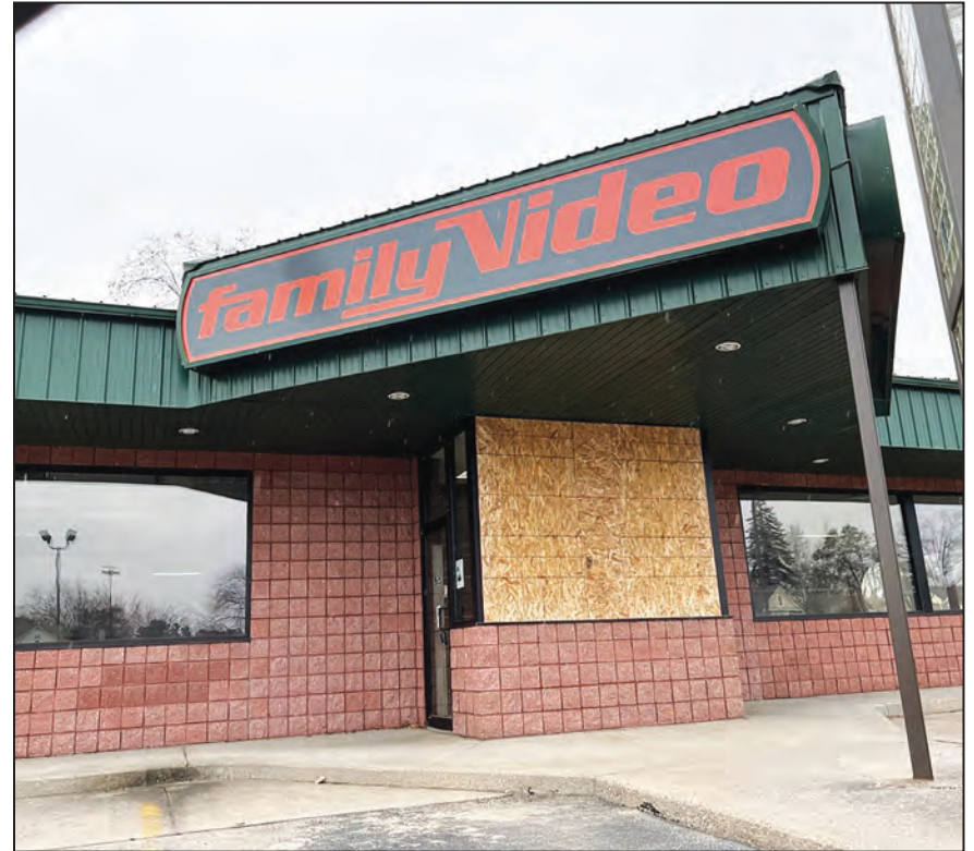
A shattered pane is boarded up at the former Family Video, 606 E. Green Bay St., Shawano. This window and others were broken on the night of Dec. 6 in Shawano. Shawano Police Department Capt. Shane Stange said that while police do not yet have a motive or a suspect, the investigation is ongoing.
