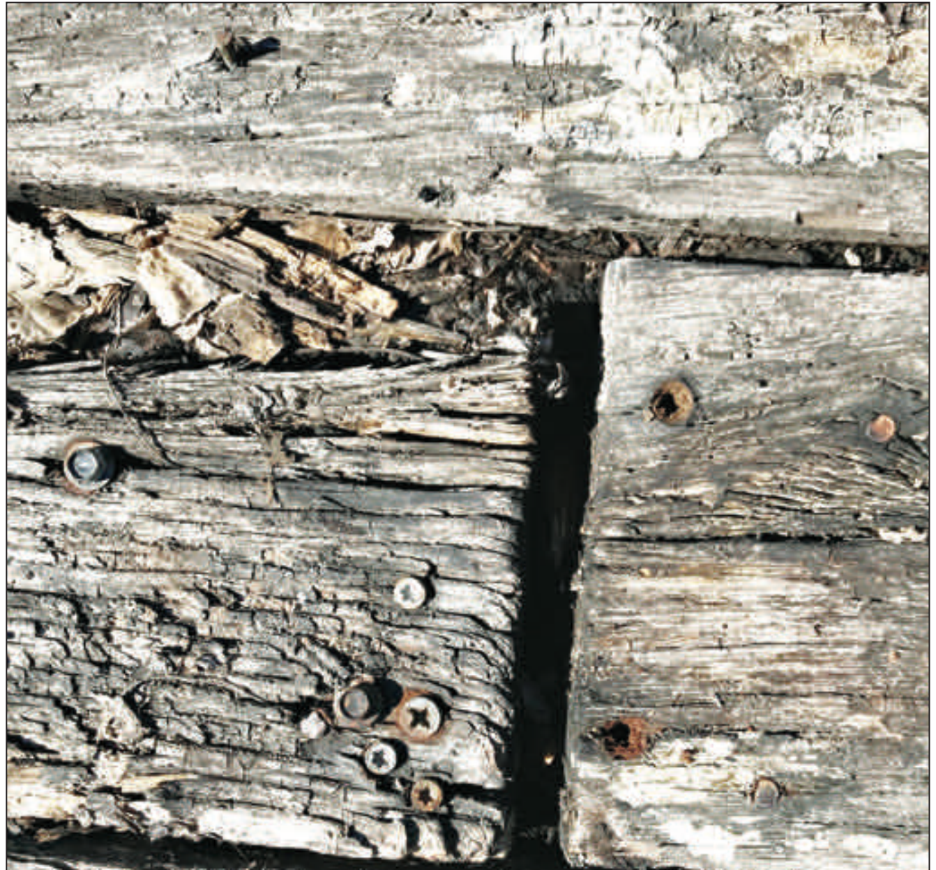
A closeup of some of the rotting boards shows bolts, screws and nails sticking out of them, posing a safety hazard for anyone crossing the bridge.
