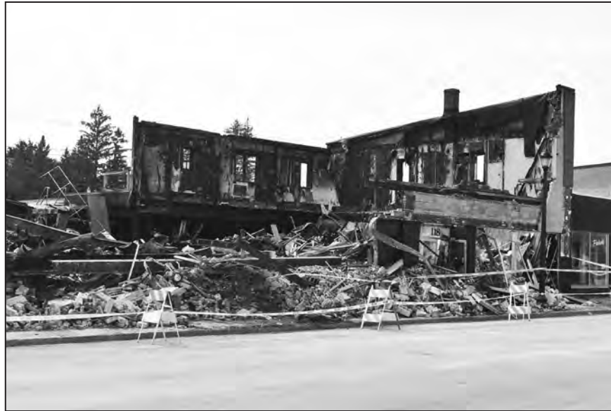
A Sept. 14 fire reduced the building at 114-118 W. Pulaski St. to rubble. People inside the structure and an attached house got out safely, but four cats were missing. No firefighters were hurt.
