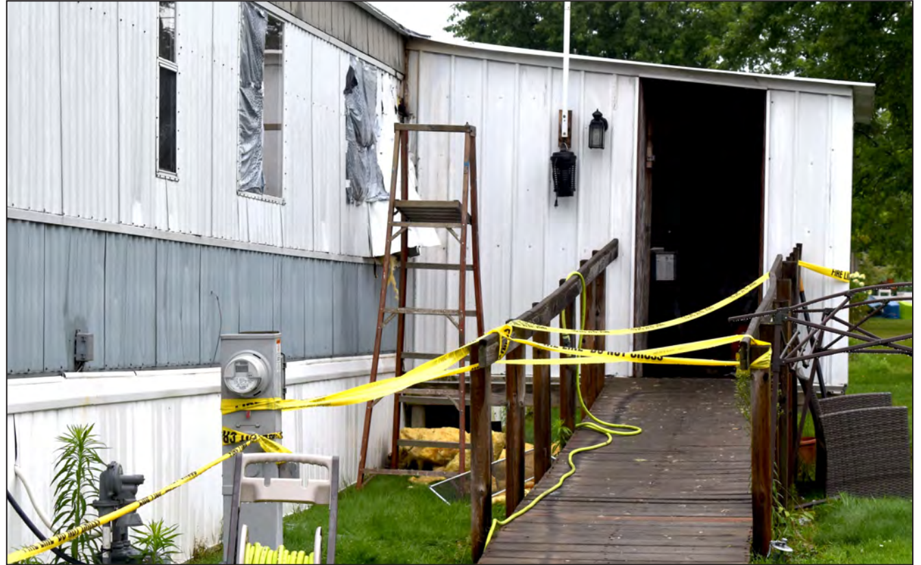
Warning tape remains in place Aug. 14 and fire damage can be seen through the front door of the mobile home at 7792 County I, Lot 32, in the Town of Stiles, after an Aug. 11 fire destroyed the home's interior.
