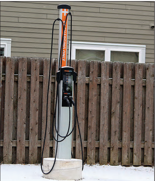
Shawano has at least two locations where there are public charging stations, including this station in the parking lot behind Naberhood Plaza. The second station is at Franklin Park. LEE PULASKI | NEW MEDIA
