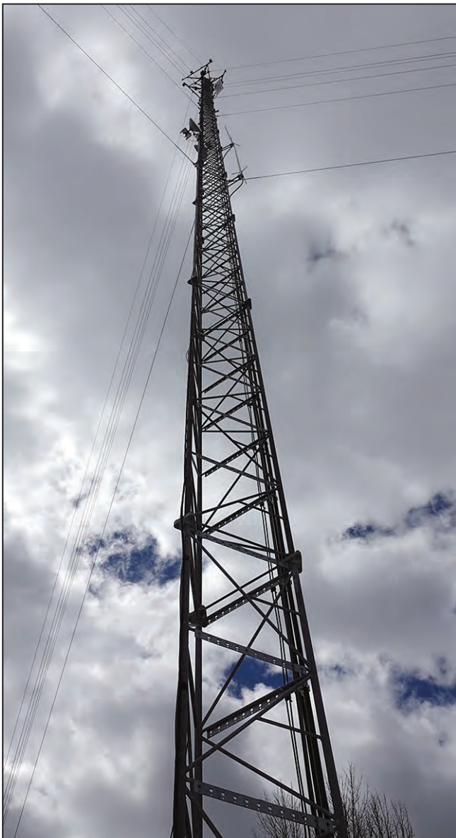
One of the next projects for Shawano County emergency management is to make the communication tower in Leopolis operational as an emergency backup. The county owns the tower, but there is no equipment on it yet. The Pella Fire Department is also interested in using the tower.
