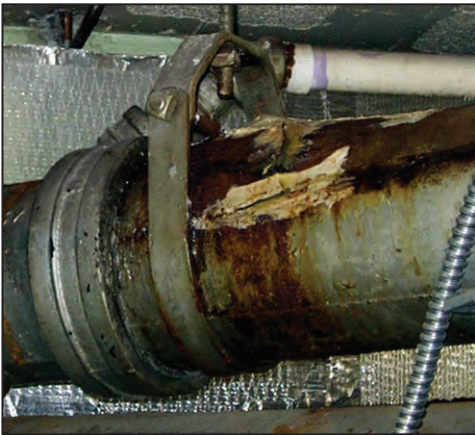
Deteriorating pipes at the Shawano County Courthouse are among the many necessary repairs cited by Somerville in its facilities assessment report completed in spring 2023. An ad hoc building committee will soon review the options for the county — whether to continue with its existing buildings in a repair and update mode, whether to significantly remodel buildings or whether to build new ones.
