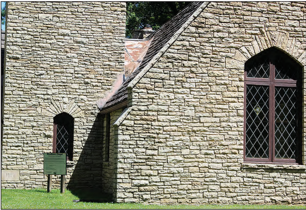
Woodlawn Cemetery's chapel is in need of some tender loving care, starting with its roof, which is missing some of the cedar shake shingles already, and the ones still attached are well beyond their shelf life. Shawano officials seek to hire Bontrager Carpentry to replace the roof.
