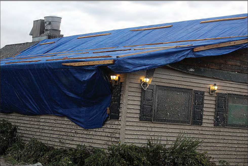
A blue tarp covers roof damage at one of the buildings for Telford Equipment Consulting Co. on July 24 after a storm came through the previous evening.
