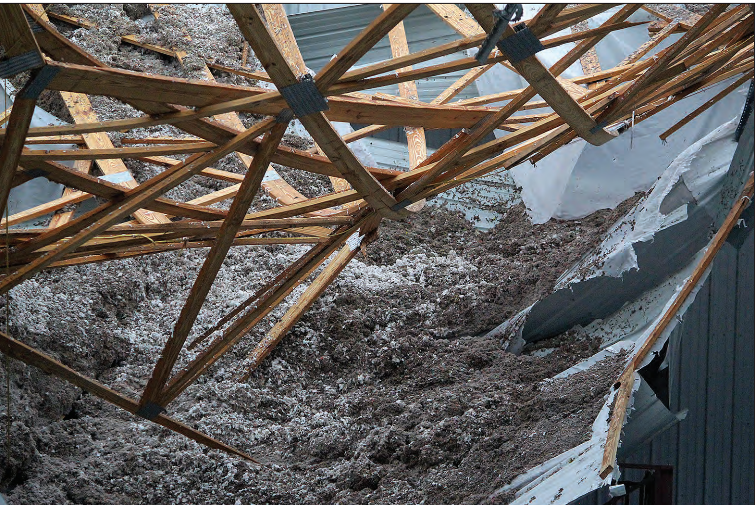
A web of wood and other materials is visible from state Highway 22 in Gillett as a building owned by Telford Equipment Consulting Co. was destroyed during a storm on July 23.
