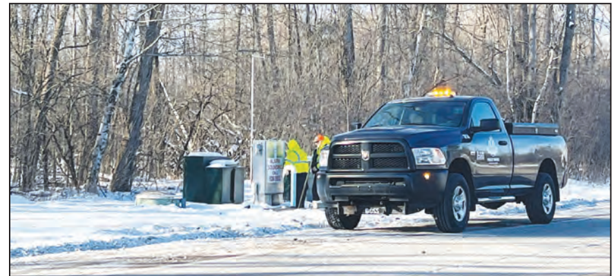
Crews with Shawano Area Fire Department work to fix a piece of equipment after a power outage caused some Shawano residents to lose power on Feb. 1. The power outage was caused by equipment failure, something that Shawano Municipal Utilities is investigating.
