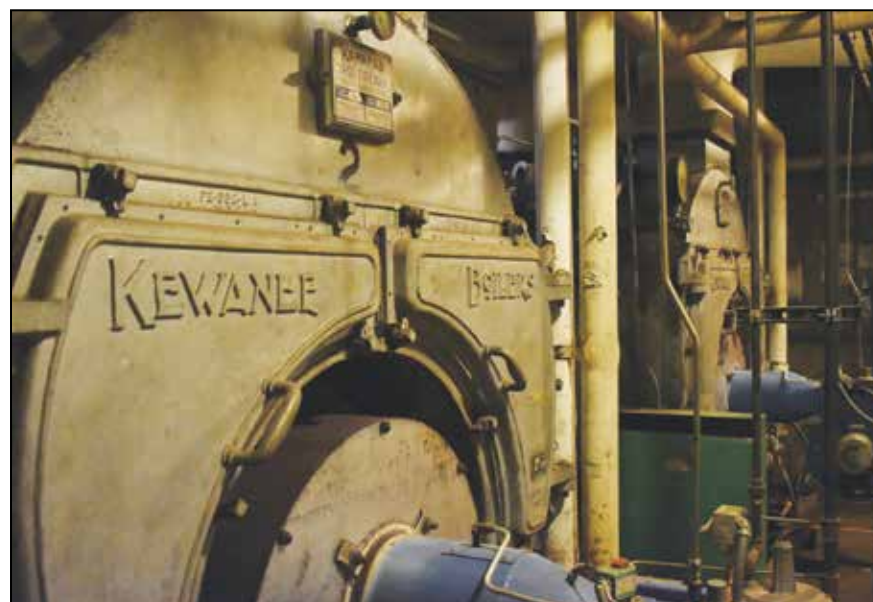
Parts for the ancient heating system at Washington Middle School are hard to find if not impossible, said Mike Bouche, buildings/grounds and maintenance supervisor.
