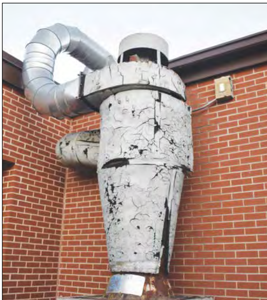
The industrial education area of Washington Middle School, built in 1983, still uses the original Stern-vent Co. exhaust collection system.
